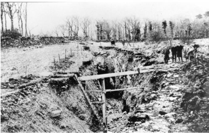
Preliminary excavation of the Goat Tunnel, looking south towards Aberglaslyn - ca. 1905 - Arch 3926.
