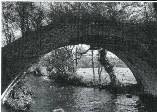
Nantlle Railway bridge near Bontnewydd. This may have been the route of the proposed extension to Caernarfon. Photo - P.Johnson
