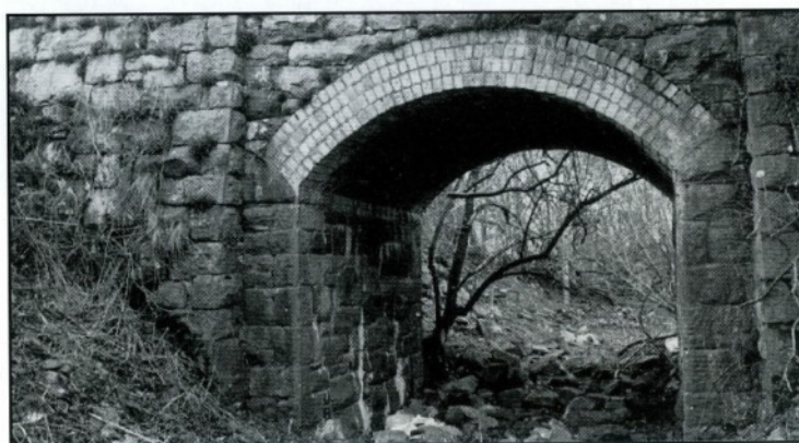
Accommodation overbridge (OB 24) east of Tryfan Junction - parapets and arch to be replaced with a concrete trough
