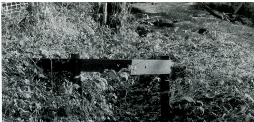
The remains of the sluice gate in the leate with the Afon Rhyd which supplied the water in the background. Photo David Allan January 2000
