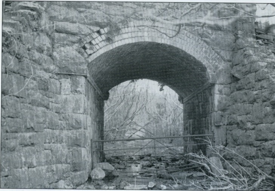
Bridge carrying the Rhostryfan road over the Bryngwyn branch. Photo D.W. Allan 1st April 1998
