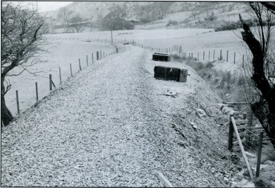
Approx point where the coaches left the rails. Photo D.Allan 4th March 2003
