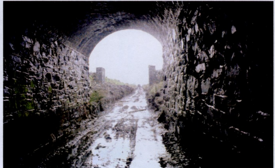
Cattle crossing abutments from beneath Pitt's Head Bridge Photo - D.W. Allan 1st May 2005
