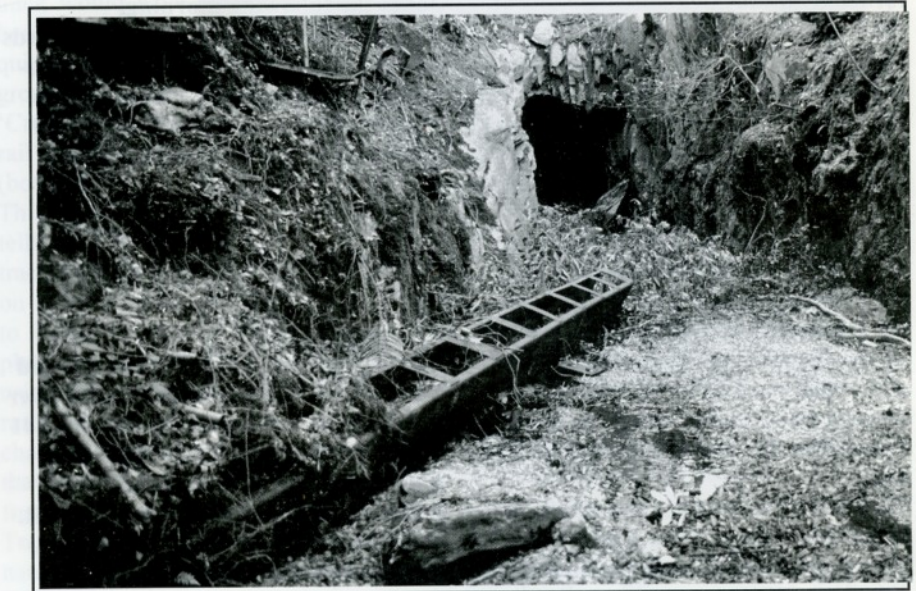
map on facing page) and must have looked impressive when functional. The 'dam wall' is of substantial stone construction topped with large slate slabs. An interesting feature is the concrete-lined overflow on each side directing water into the aqueduct. One wonders whether these overflows were incorporated in 1922/3 to prevent surplus water cascading onto the trackbed, which up to until then wouldn't have been used as a railway. But where was the source of water to maintain the reservoir's level? Plans produced for the proposed NWNGR's Beddgelert Extension - the terminus of which was planned to be a field away from the reservoir - and the 1913 O.S. map provide the clues. From the inlet a 60-yard ditch parallels the field wall to a point where three fields meet. Here the 'feed' turns through 90 degrees and one suspects that it is here that the original watercourse was diverted to provide some of the reservoir's water. The stream then crosses a field to a further intersection of fields where The Goat aqueduct lies forlornly at the side of the Goat Cutting in April 2005 - D.W. Allan
