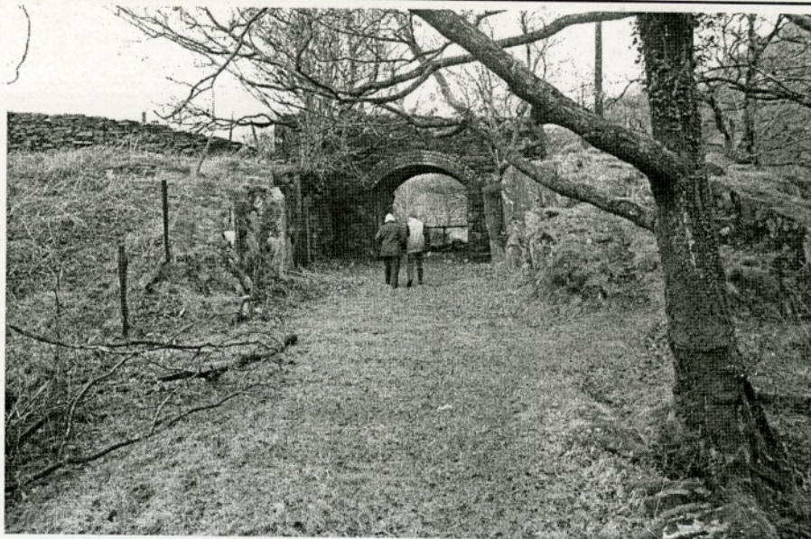
Pont Cerig y Rhyd bridge - this is roughly where the coal wagon would have been when sighted by driver Beaumont when he was 15 yards the far side of the bridge.
