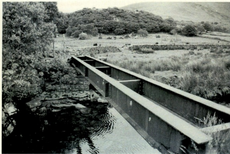
Line of tramway from the WHR near Tan-y-Ffordd to Garreg Fawr Slate Quarry. The girder spans the Afon Gwyfrai.
