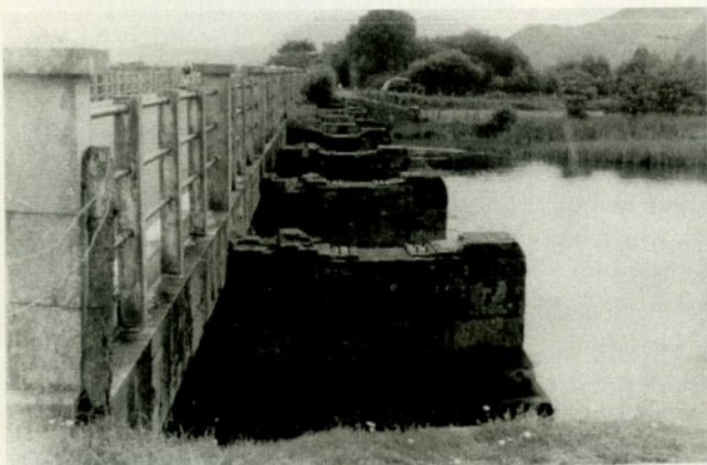
Pont Croesor:- Detail of stone piers showing concrete plinths & holding down bolts
