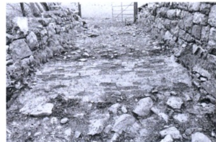
Bricks show through the road surface of the accommodation bridge between Tryfan Jct & Tan-yr-Alt
