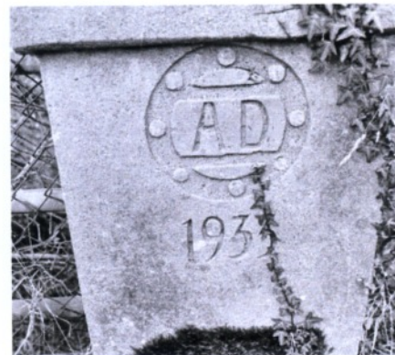
Engraving commemorating the 1933 rebuild of Wernlas Ddu road bridge destroyed by Gwynedd County Council when the parapets were upgraded
