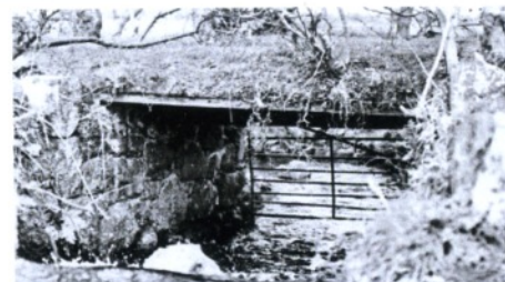
Doubtful support for the trackbed as it crosses the Afon Rhydd
